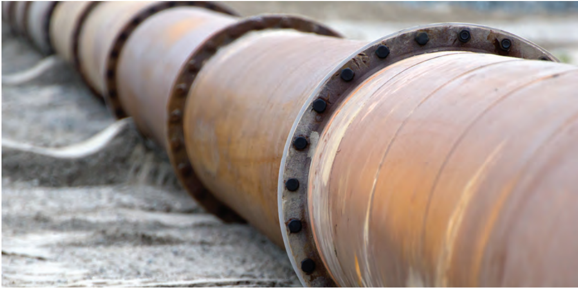
Rusty pipeline. Credit: Shutterstock
